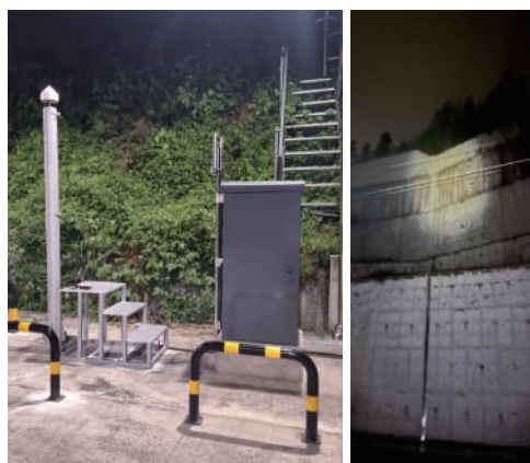
Railroad facility monitoring
